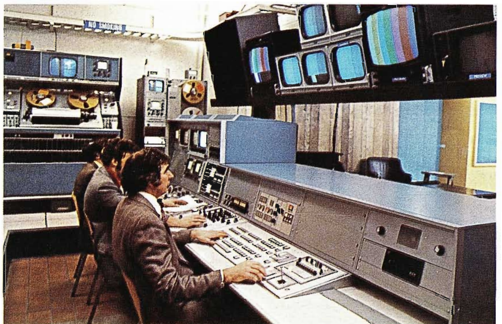
The Control Room is adjacent to the studio. All of the racks and equipment are mounted on a computer floor, making for a neat, efficient installation. Production is normally handled by a three-man control room crew: A Director who does his own switching. One man operates the TR-70 and TR-60 VTR's (both are used in original recording) from the remote panel of the Time Code Editing console—and also rides audio levels. The third crew member shades the TK-44B's via joy stick remote controls.
